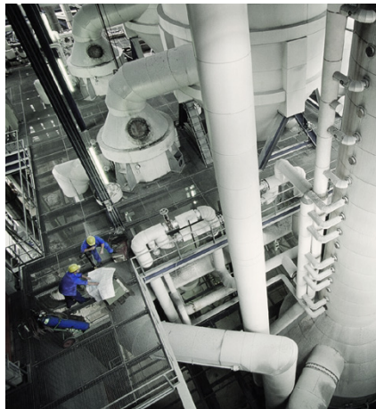
Optimal integration: Minebea Intec's weighing technology fits perfectly into Salinen Austria AG's production halls.
