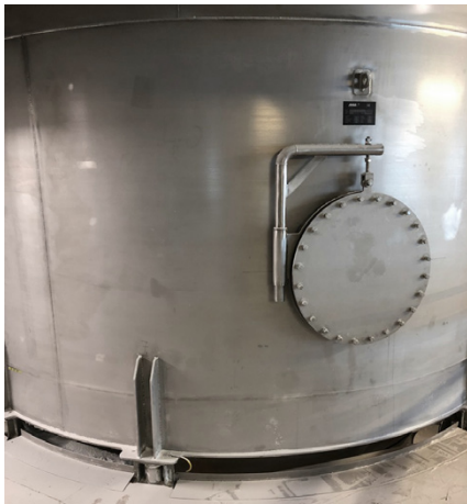
Specialist advice: due to the large capacity of up to 150 metric tonnes, eight load cells were installed in each tank.
